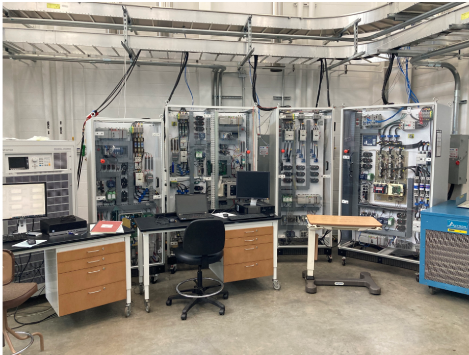
Figure 3.13: photo of the High Bay Lab microgrid in Wisconsin Energy Institute
